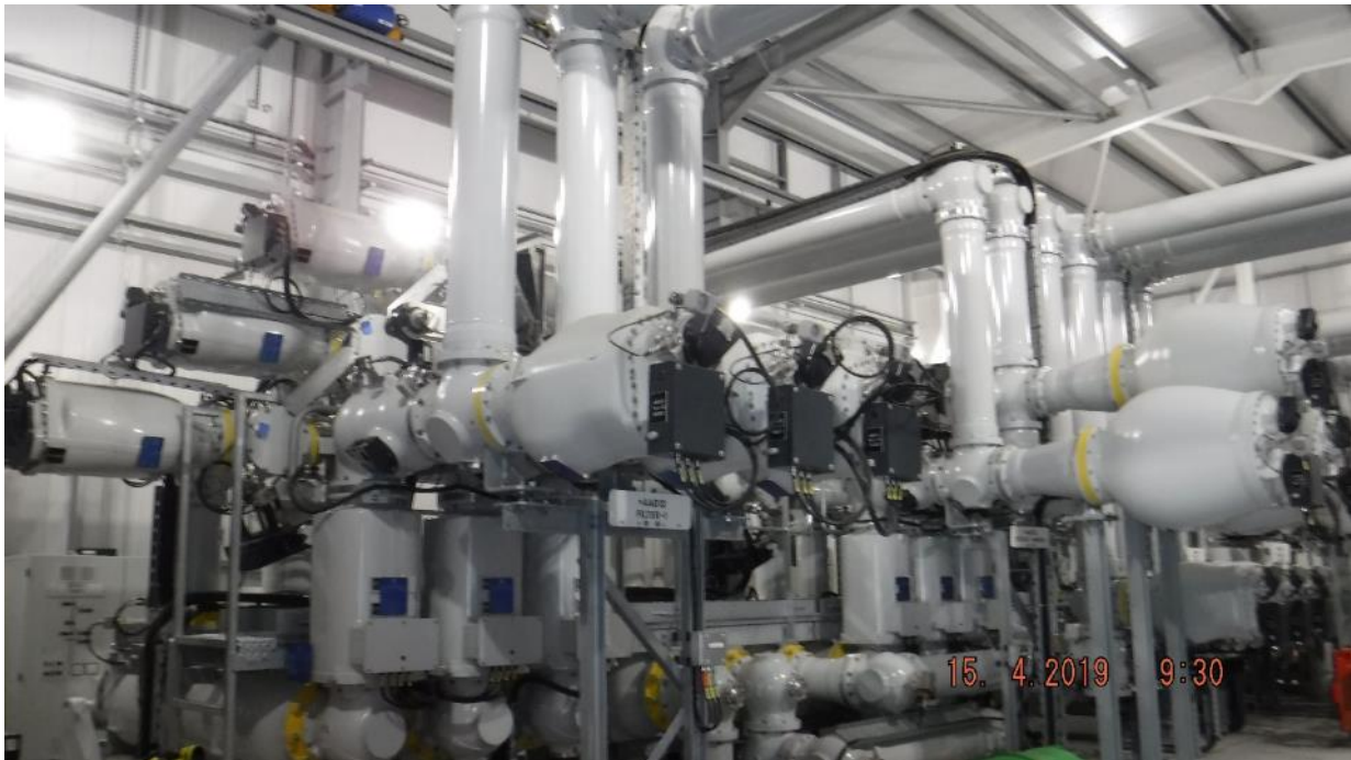
Plate 2.9 Electrical Equipment Contained within the Onshore Substation (example taken from East Anglia ONE substation)
