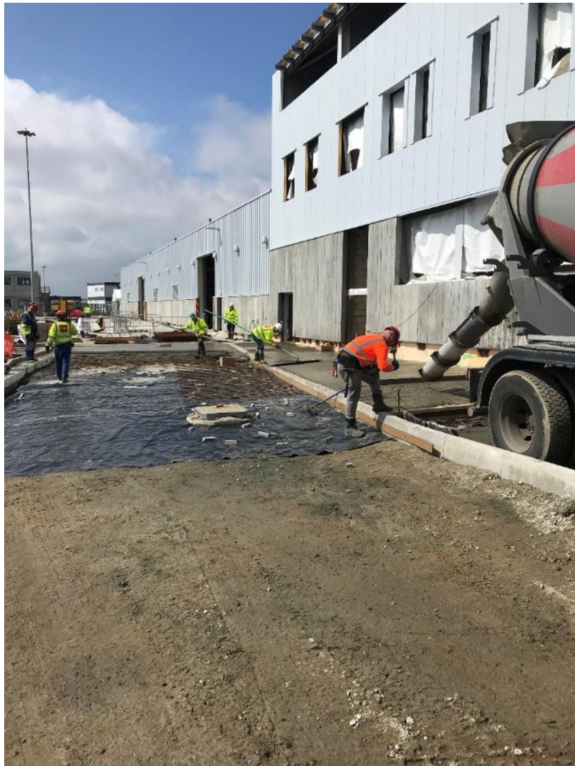
Plate 2.13 Construction of Substation Operational Access Road (example taken from East Anglia ONE substation)
