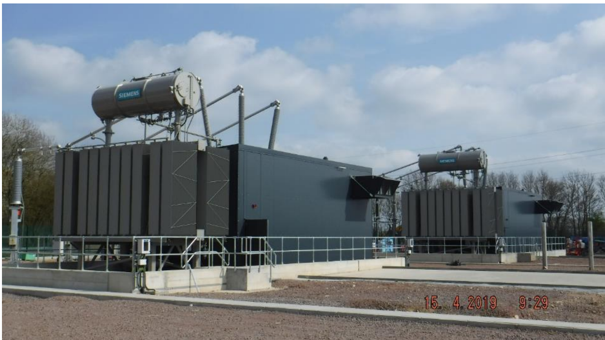
Plate 2.10 Example of Shunt Reactor Building to House Reactive Compensation Equipment (example taken from East Anglia ONE substation)
