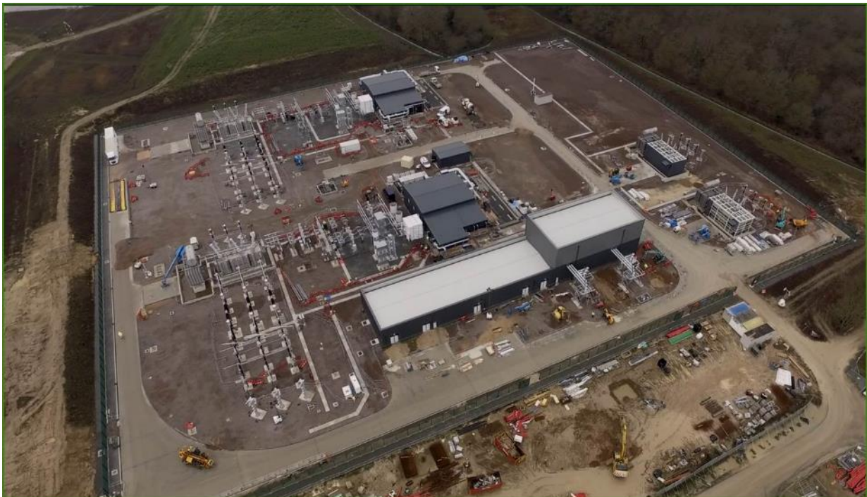
Plate 2.12 Example Layout of the Onshore Substation (example taken from construction of East Anglia ONE substation)
